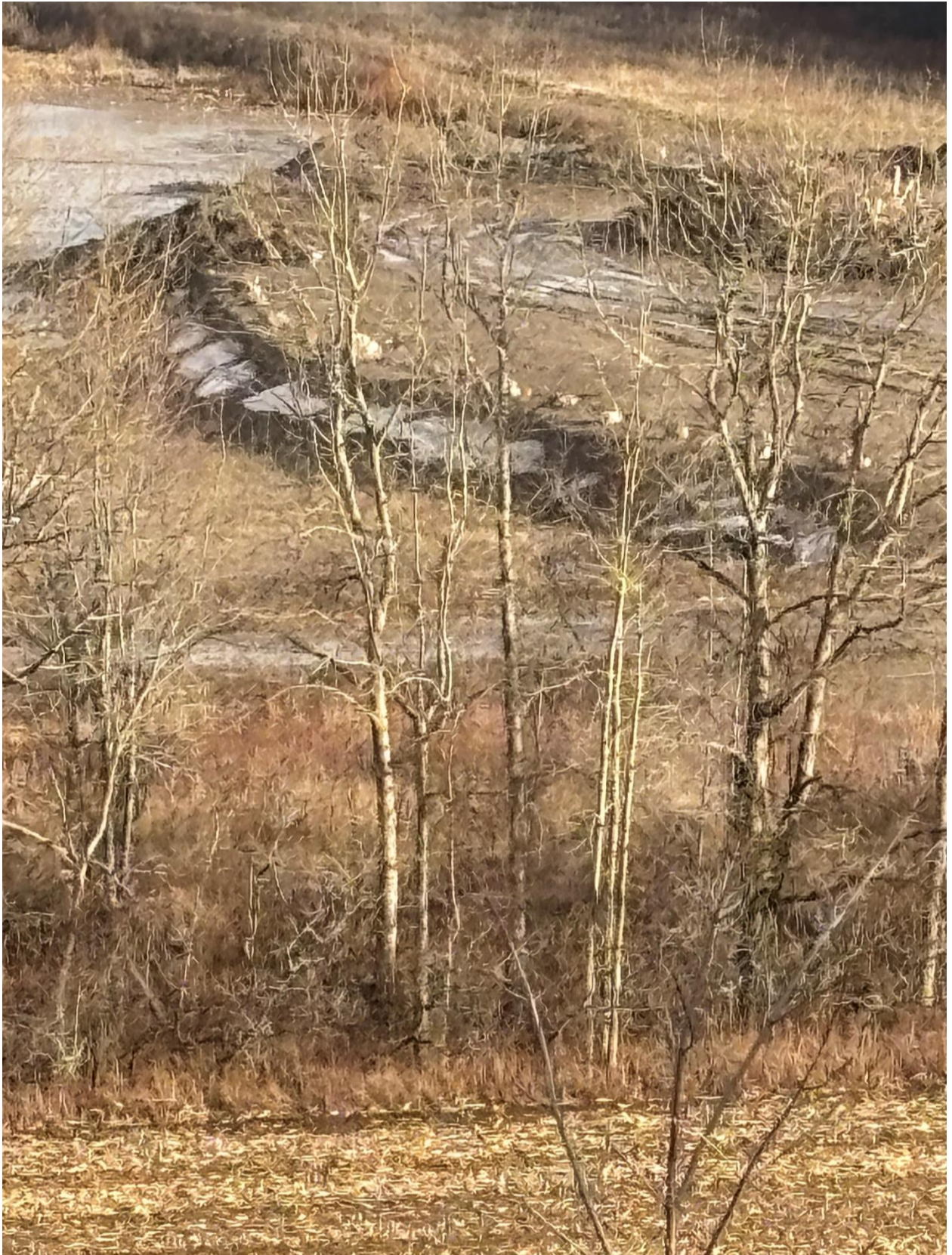
This picture was taken December 17, 2024 and shows the area in the pit that is being filled.
