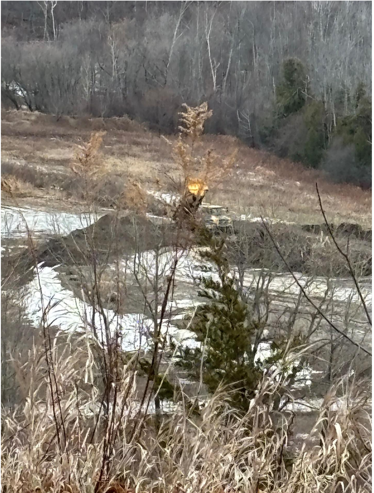
This picture was taken December 16, 2024 and shows the dumping of fill into the subject area next to and into the Environmental area. Dump trucks and Quarry Trucks full of fill from a pit located on Little Lake Rd were brought in, piled and deposited into this area.
